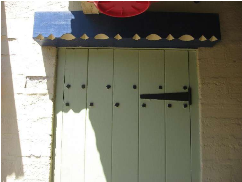
Detail of studded service door. Note carvings on lintel. (Author Photo. July 2023)
