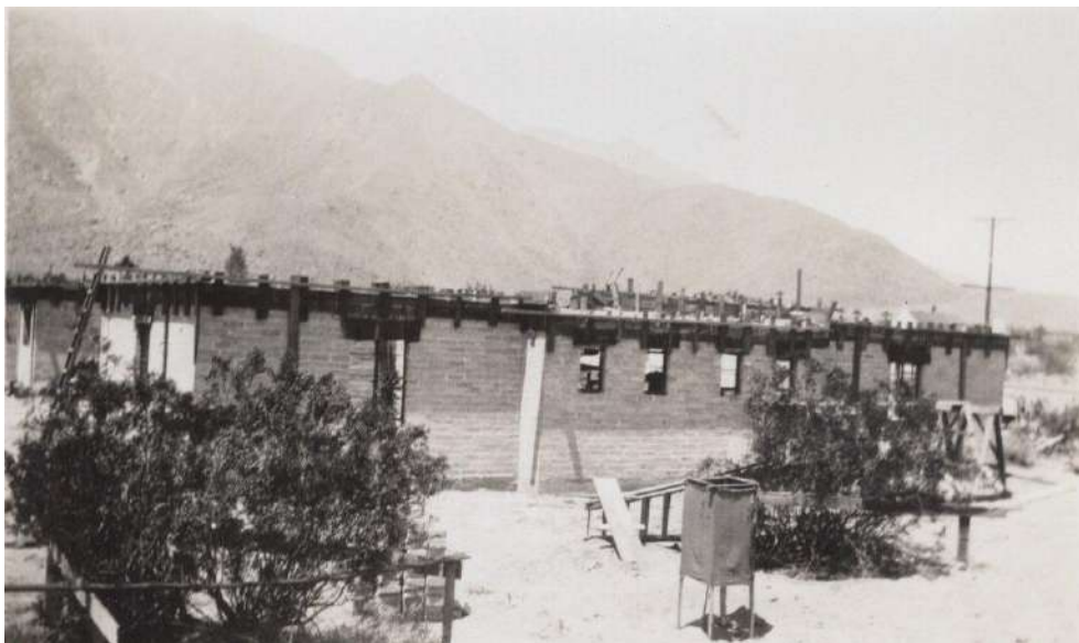
Construction photos ca. late 1931. Top view looking northeast. Bottom shows east façade. Note, quartet of windows.
